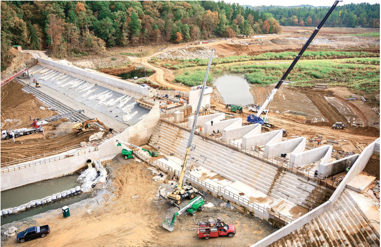
The rehabilitated Lake Williams Dam features a labyrinth weir and spillway. Once full, the reservoir will include 'turtle island' and aquatic habitat features.
